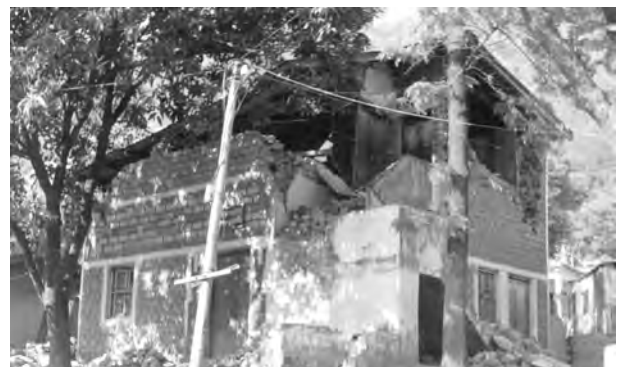
Figure 6.1 : A Damaged Building Due to an Earthquake
