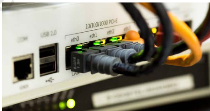
Figure 10.12: Cables connected to a network switch
