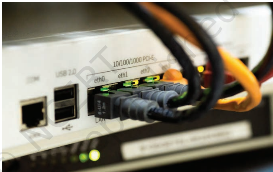
Figure 5.9: Cables connected to a network switch
